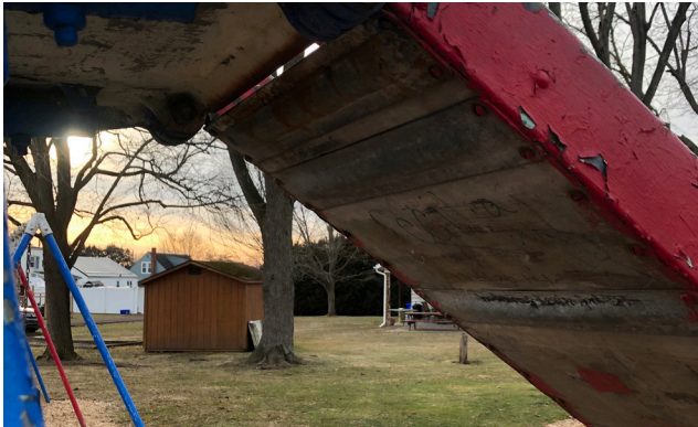
A dangerous gap at top of slide could catch clothing and cause choking. The play element also has flaking paint and rust.
