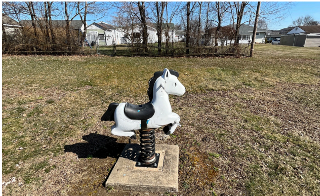
Exposed concrete footing with sharp edges within fall zone can cause injury. There is a lack of safety surfacing.
