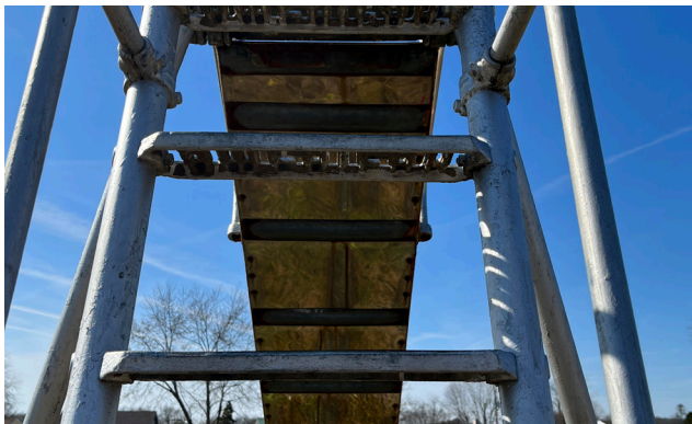
Exposed fittings can catch clothing and cause falls or injury. The play element also has flaking paint and rust.
